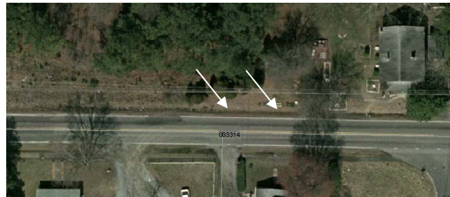
Evidence of Drainage Ditch Interfering with Sidewalk Construction (Dearborn Av).
