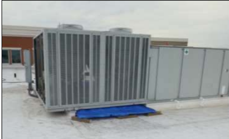
Figure 2. Containment tarp and PVC pipe structure shown underneath HVAC unit prior to field blank collection at Site 3.
